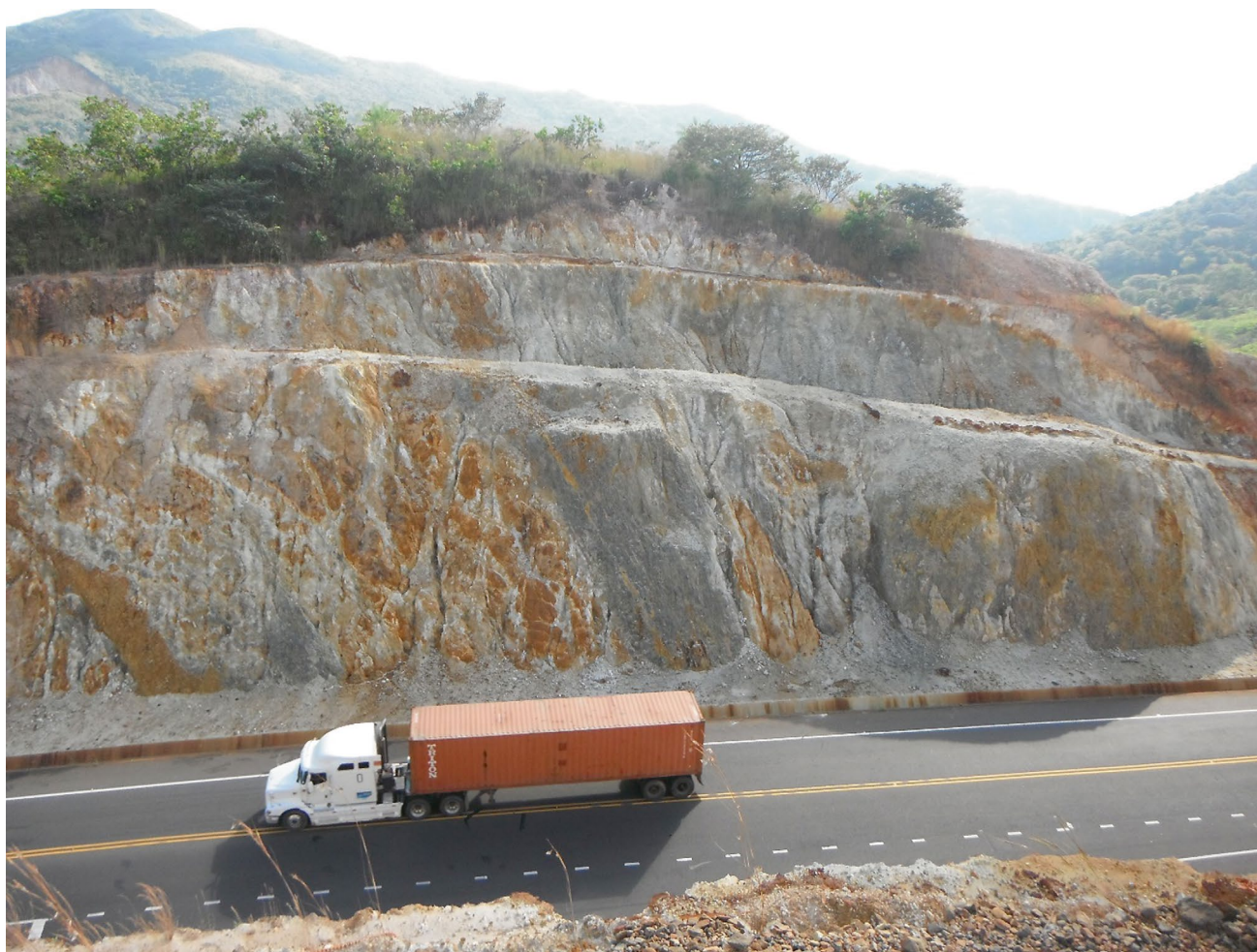
Fig. 12.5 Road cut in Route 27, km 47. Intense hydrothermal alteration and terracing to stabilize the slope are observed
